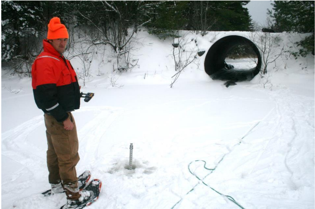
Figure 5. Photo identifying location of the plunge pool (8.7 feet deep) relative to the culvert.
