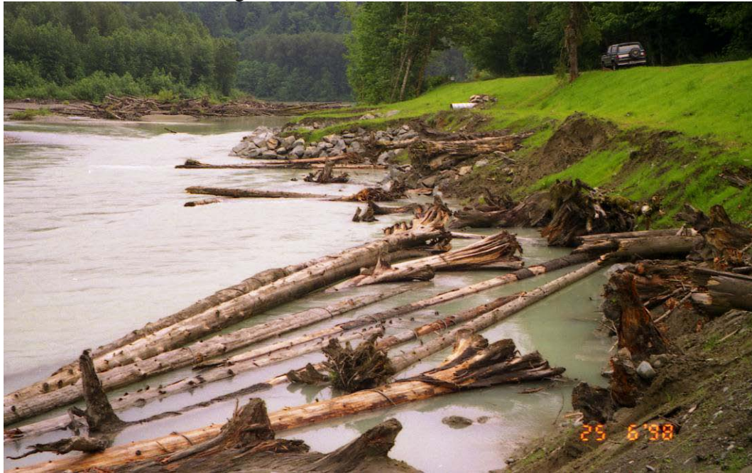
Figure 6. Large wood tethered on long cables to large drilled boulders (Sauk River side channel near SR 530, Skagit Co., WA).
