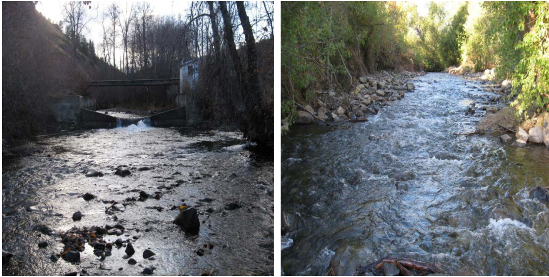
Figure 6. Diversion weir (left) replaced by roughened channel / constructed riffle (right). North Fork Ahtanum Creek, WA.
