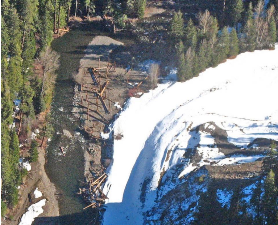
Figure 15. Floodplain wood placed on a constructed bar to roughen the former active channel where it previously abutted a rip-rap roadbed. The logs are braced against and attached to vertical log pilings (Klickitat River, WA, Inter-Fluve, Inc.).
