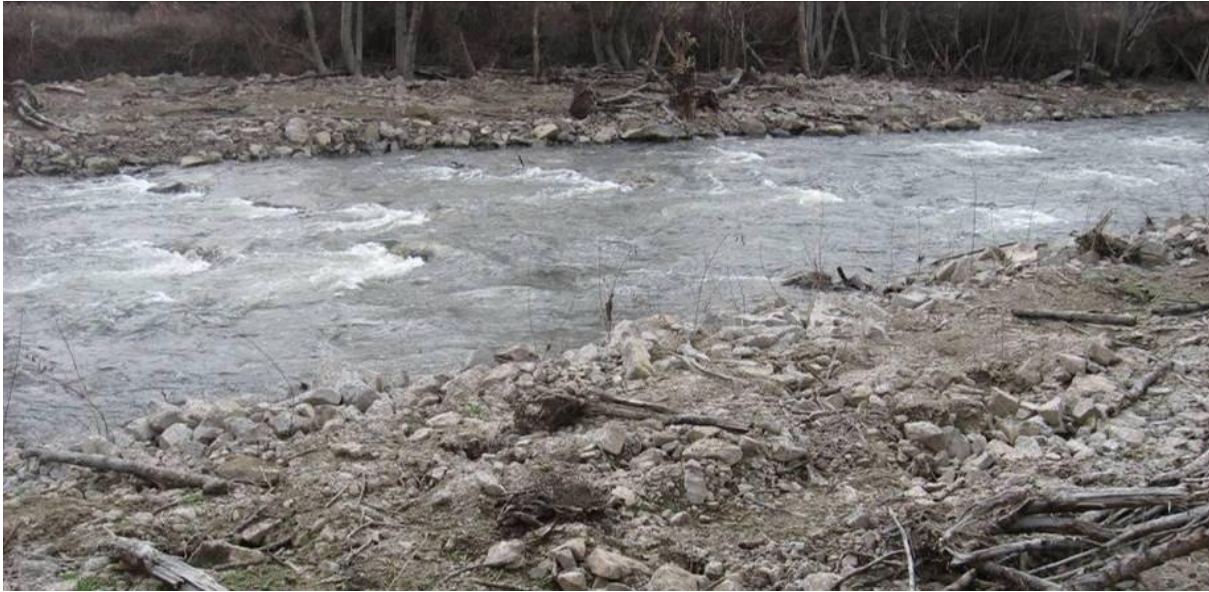
Figure 11. Roughened channel / constructed riffle constructed following dam removal (February 9, 2010). Source: Inter-Fluve, Inc.
