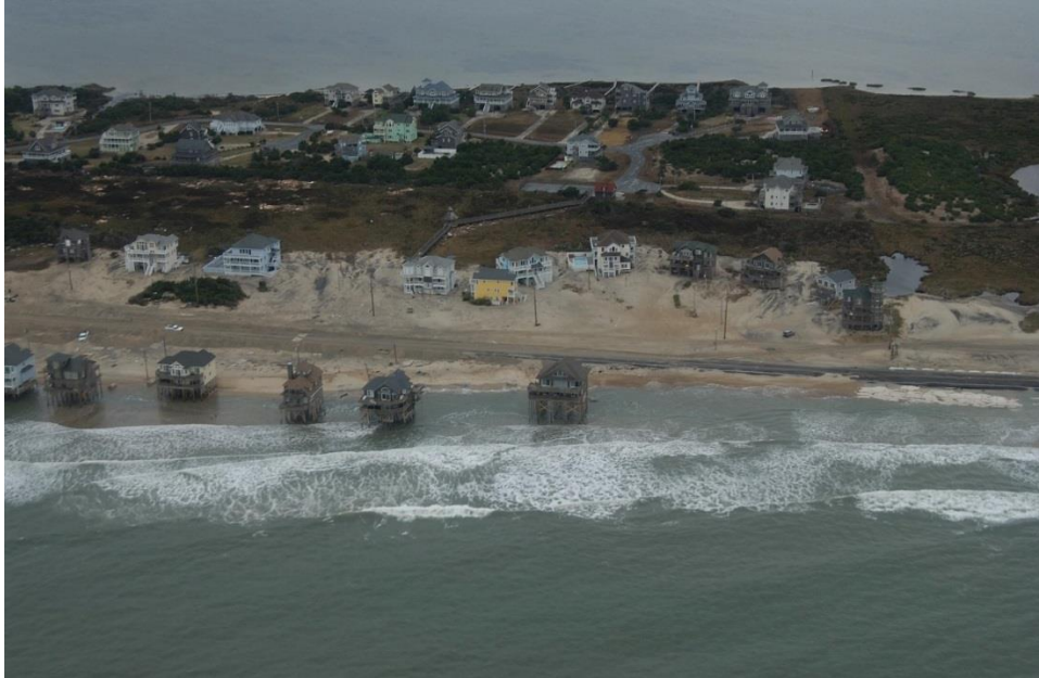
Figure 8. Hurricane Sandy deposited overwash in Rodanthe, NC, creating overwash fans in a developed area along NC 12. NC 12 is buried by overwash on the left side of the photo and undermined by erosional scour at the right side of the photo, where sandbags had been placed to protect the roadway. The sandy beach habitat has been modified by the storm to retreat landward and to remove any dunes. Image from USGS (2015) dated November 4, 2012.
